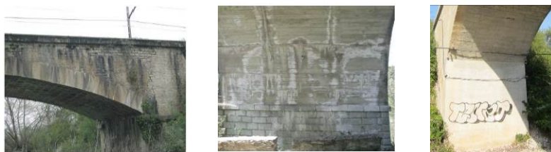
Fig. 1. Stains, crusts, efflorescence, vandalism, etc.
