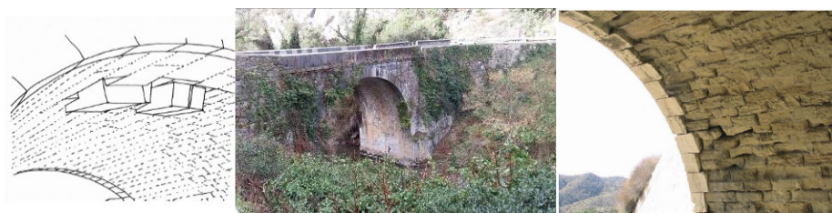
Fig. 2. Loss of material from joints and pieces, vegetation, previous interventions, etc.
