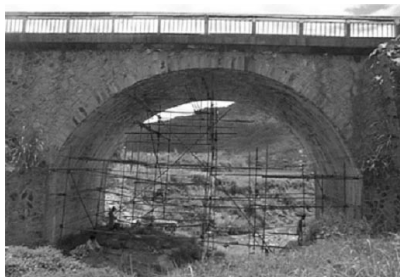
(a) Under reinforcement
