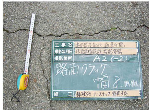
Figure 4: Cracks on Asphalt Pavement
