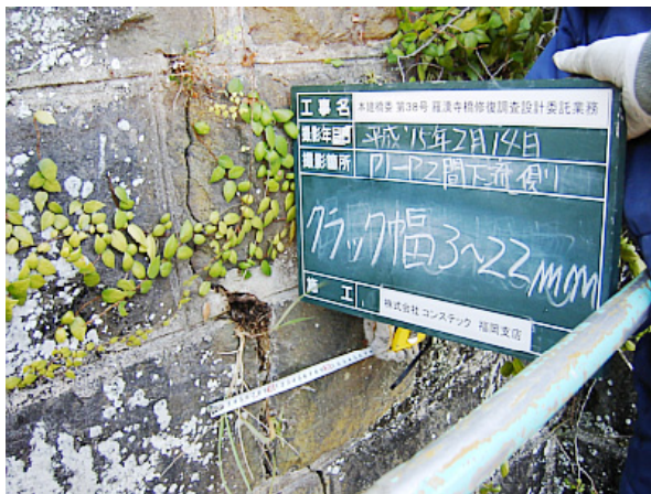
Figure 3: Cracks on Spandrel
