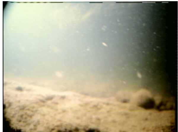
Figure 13: Gap between Pier and River Bed
