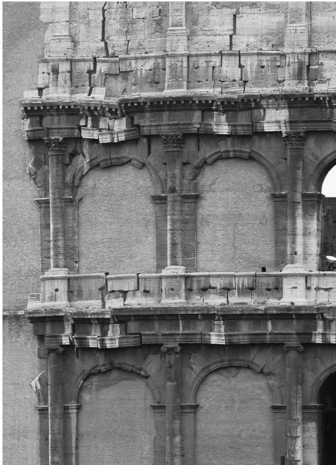
Figure 1: Damages preserved in the restoration work by Stern (1814-1820).
