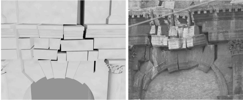
Figure 8: Detail of the key voussoir of the third level arcade. Left: three-dimensional simulated mechanism. Right: actual damaged state.
