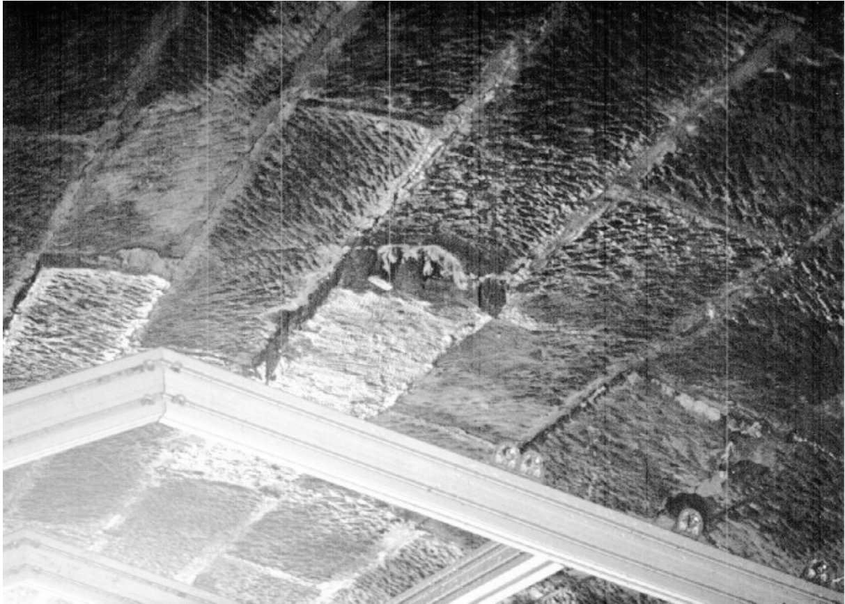
Figure 2 Dropped stones near the inner face of the spandrel
