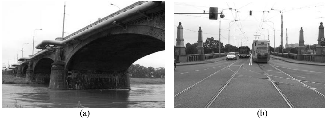
Figure 2 : Osobowicki Bridge: (a) main spans with visible pipeline system, (b) bridge deck with the usual traffic.
