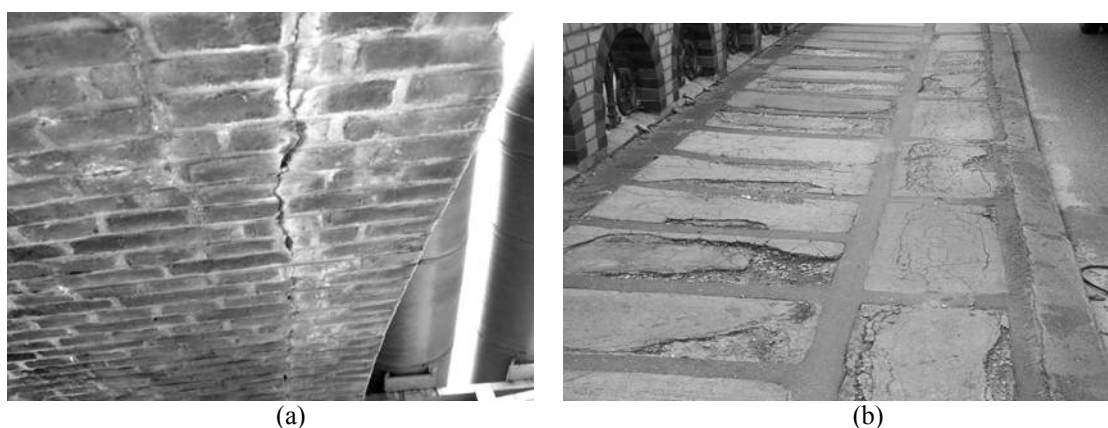
Figure 5 : Typical defects: (a) longitudinal cracking along the edge of arch barrel: (b) losses on the pavement surface.
