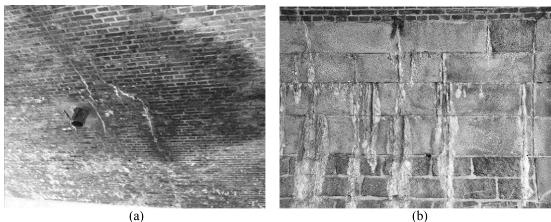
Figure 4 : Typical defects: (a) longitudinal cracking and moistening of arch barrel: (b) leaching at arch barrel springing.
